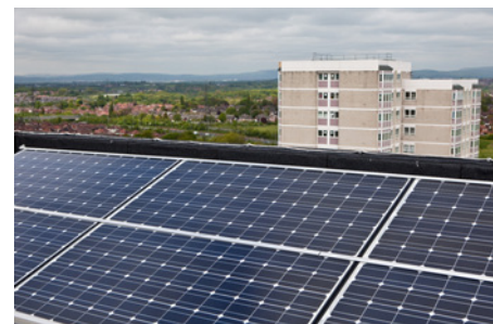
Northwards' installations include solar PV on blocks of flats to power communal lighting.
