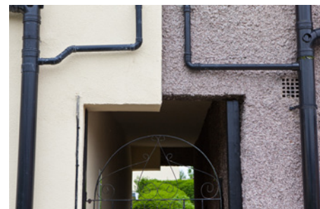
Solid walls are insulated externally as can be clearly seen on the building on the left.
